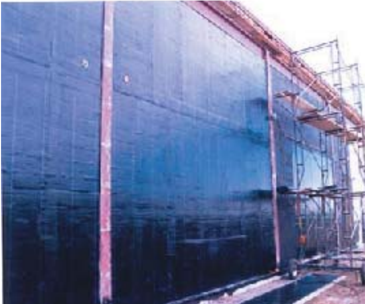
Figure 1: Does your air barrier consistently look like this? It should !
