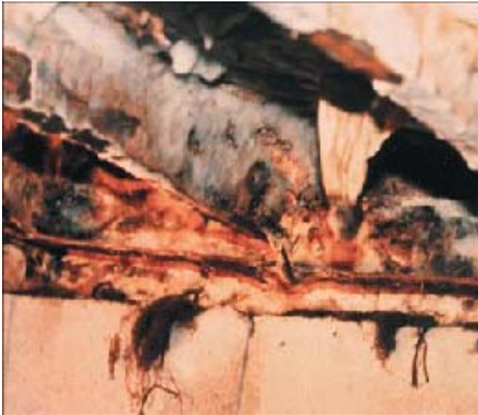
Figure 2: Damage to Wood from moisture
