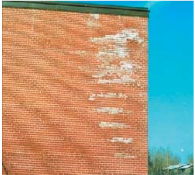
Figure 3: Visible Signs of a Building Envelope in Distress from the Exterior
