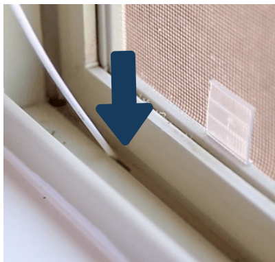
Interior weep holes.
