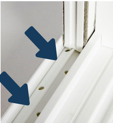
Interior weep holes.
