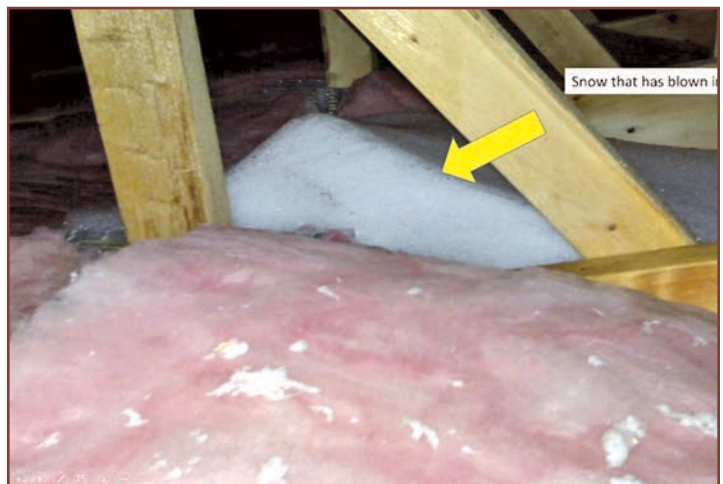
Figure 3. Snow in attic.
