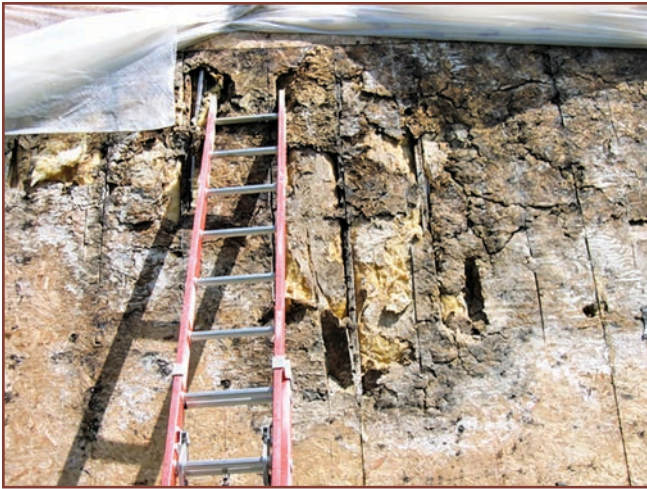
Figure 9. Rotten, five-year-old walls.
