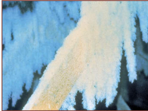
Figure 7. Frost in attic.
