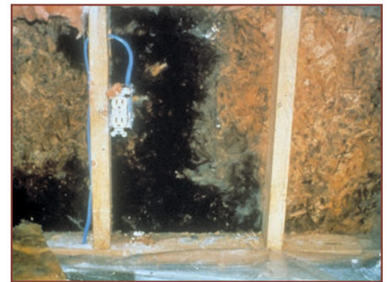
Figure 8. Mold on sheathing.
