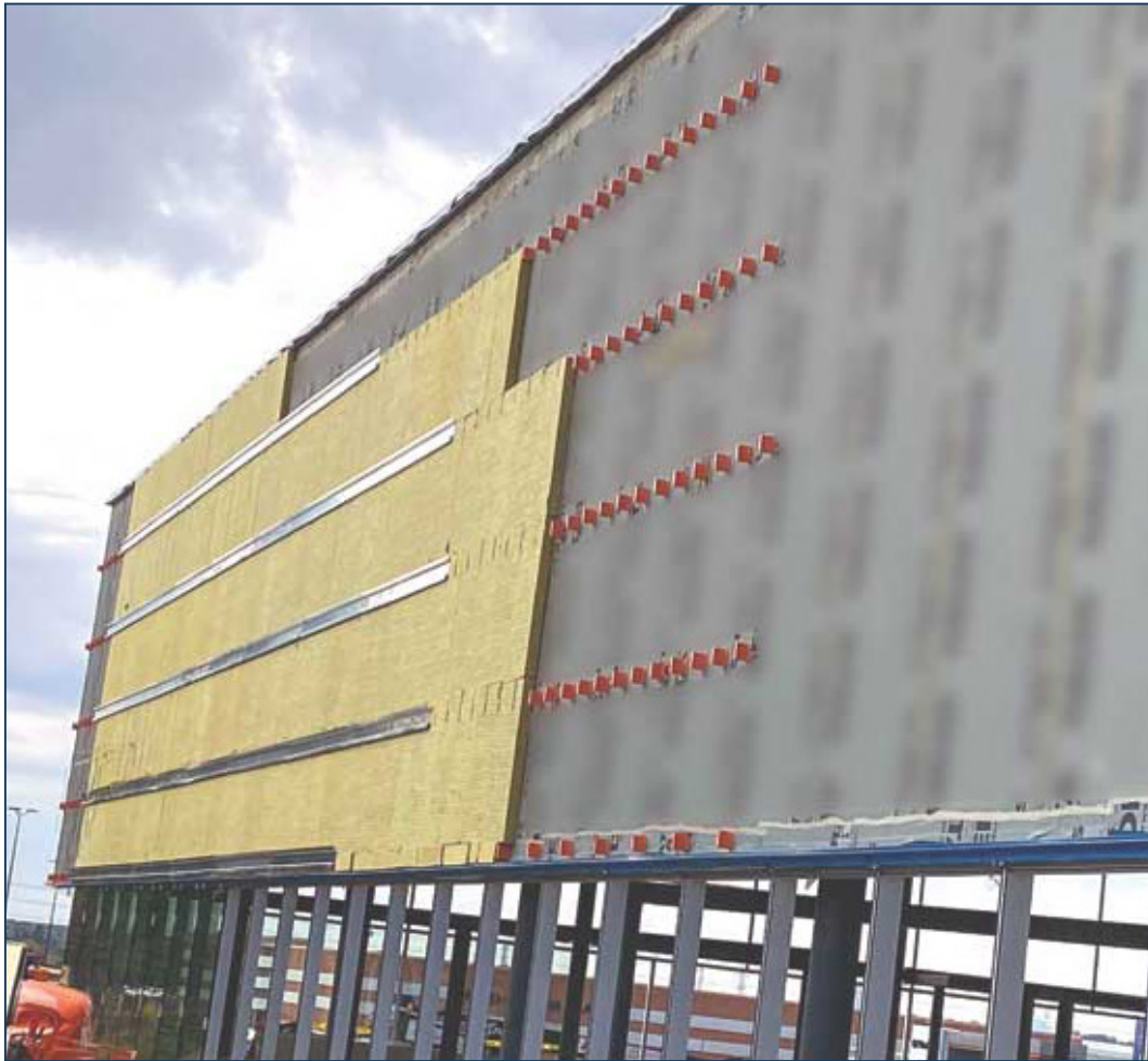
Preventing dangerous moisture from getting into buildings requires a continuous water-, air-, and weather-tight barrier. Photo courtesy Weis LGA Architects and Gaydon Contractors.
