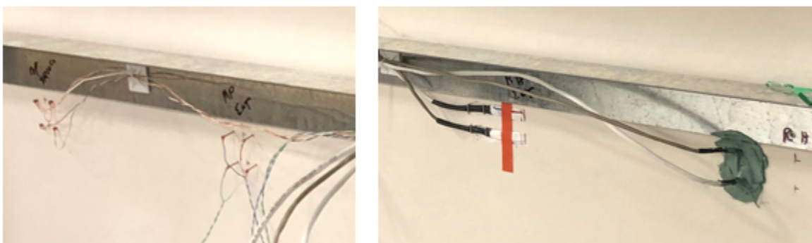
Figure 6: Moisture pin probes (left) and capacitance-type RH sensors (right) are embedded in the exterior gypsum sheathing.
