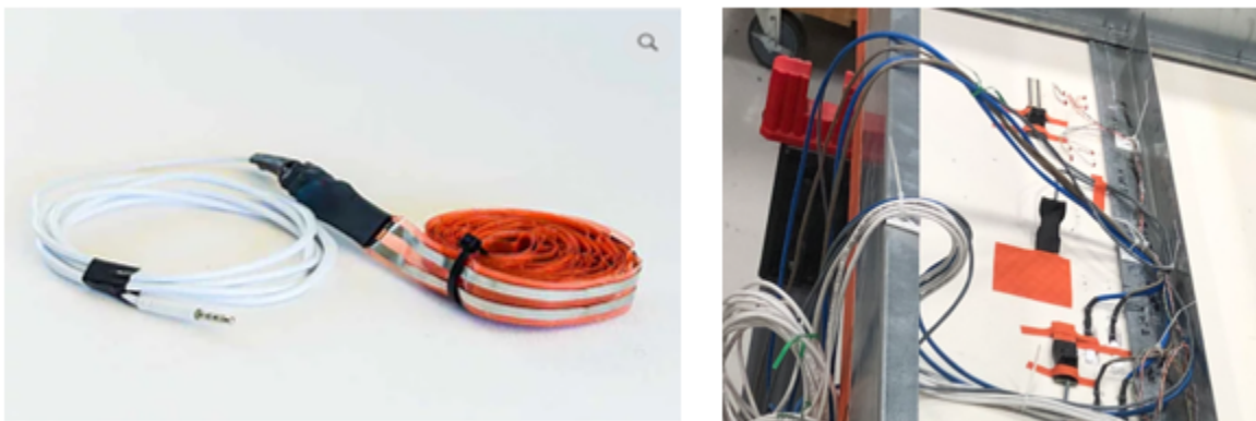
Figure 5: SMT electric sensor tape was placed horizontally on both surfaces of the exterior gypsum sheathing.
